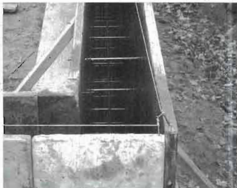
Fig. 5.2: Strong forming is critical to pouring concrete walls. Note frequent cross ties that keep the forms from spreading.
