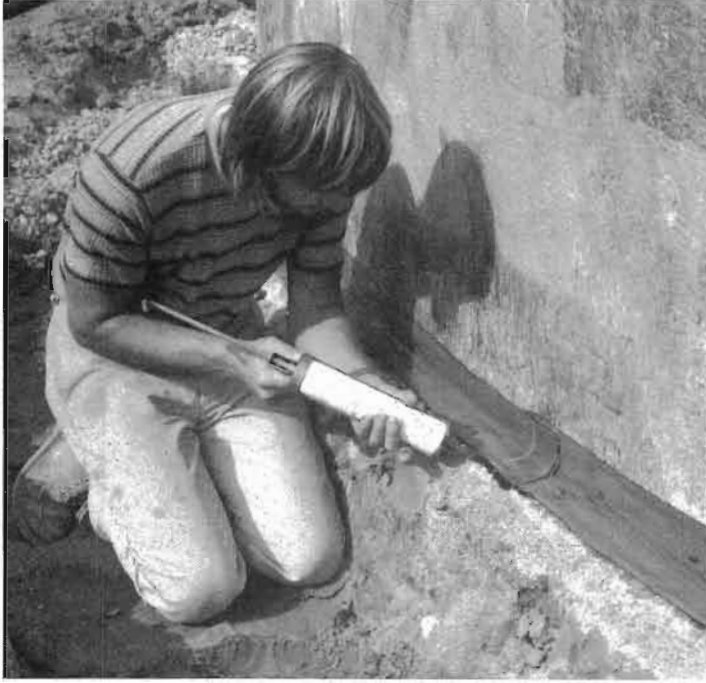
Fig. 7.1: The important waterproofing detail where the wall meets the footing is sealed with a strip of Bituthene®. Here, I am caulking the freshly cut edge.
