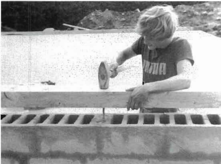
Fig. 5.12: Wait for the anchor bolts to set in the concrete plugs in the block cores. Then, locate the holes by laying the plate on the anchor bolts and whacking once sharply with a heavy hammer.
