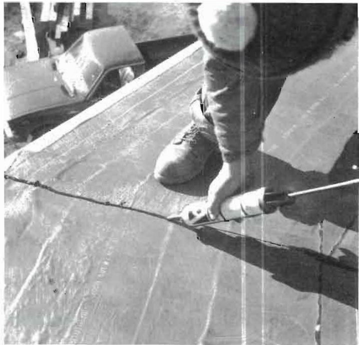
Fig. 7.9: Exposed cut edges must be sealed with a compatible caulking. After applying a bead of caulk, use a butter knife to create an edge that looks something like the factory edge. Tip: bend the last inch of a non-serrated butter knife just a little bit to make an excellent tool for this purpose.
