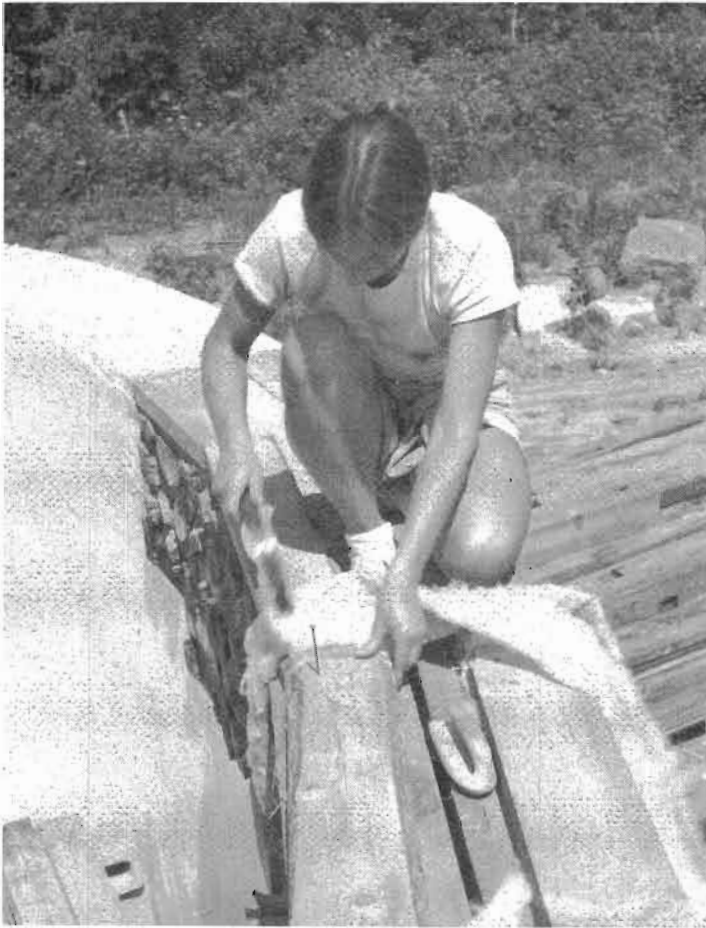
Fig. 6.16: Jaki fastens the wooden plates to the four-by-eight window lintels with 16-penny (3/4-inch) nails. To stop draft, she has installed a strip of fiberglass insulation between the plates and the lintels.
