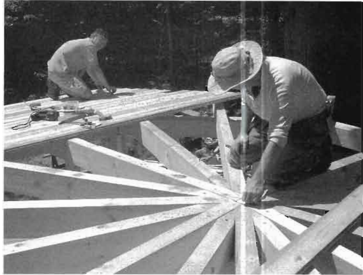
Fig. 6.18: Planking the roof at the Stoneview guesthouse was a lot like doing the Earthwood roof. Here, we snap a line on the planks, but directly over the middle of the 4 × 8" rafters. Next we cut off all the "waste" at once with a circular saw.
