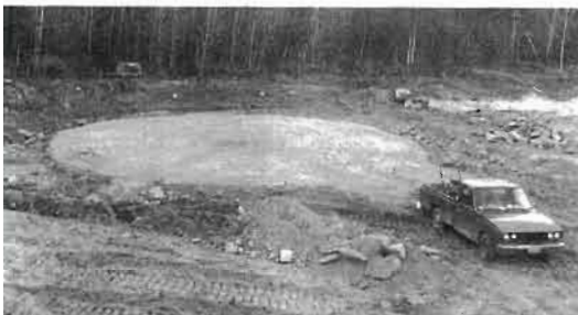
Fig. 3.6: A view of the finished sand pad at Earthwood. The pad extension near the truck is for the greenhouse.
