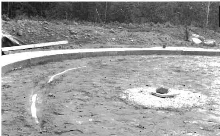
Fig. 4.4: did a good job of spreading and “backblading” the sand to a consistent four-inch depth. The next day, we hired a power compactor to tamp the sand. Jaki watered the sand with a watering can – we had no running water on site – while I ran the machine. Hitting each square foot three times with the compactor results in a solid base for the concrete floor.
