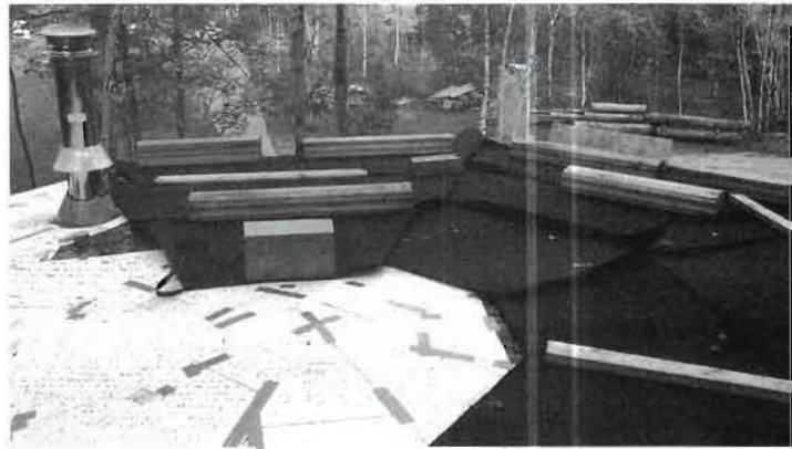
Fig. 8.6 (below): Trapezoidal sheets of Enkadrain® 361SR composite drainage are placed over the plastic, with the filtration mat uppermost. No, we haven't forgotten the plastic sheet. You can see it poking out here and there. A large centerpiece of plastic will be tucked under the Enkadrain® before it is covered with earth. Heavy wooden blocks keep everything in place until the earth goes on.
