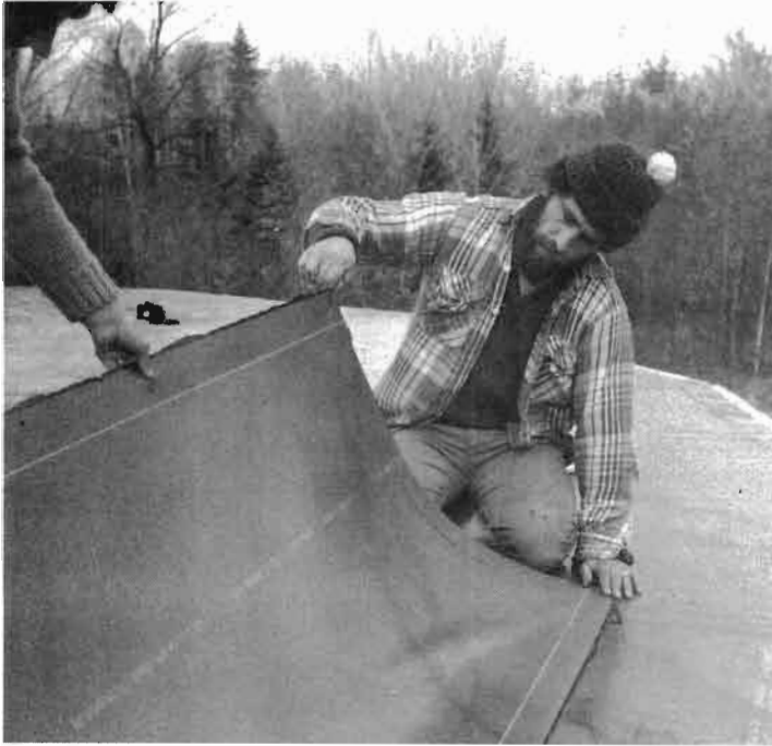
Fig. 7.8: Later, when the adjacent sheets of the same course are installed, they too should extend onto the next facet by three inches, giving a six-inch lap where two facets meet. Normally, a 3-inch lap is sufficient with Bituthene® 3000 and 4000 membranes, but you want extra protection where facets come together, pressing hard onto three inches of solid wood on each side of the crack. Apply the lower edge of the Bituthene® first, using the white line on the previous sheet as a guide.
