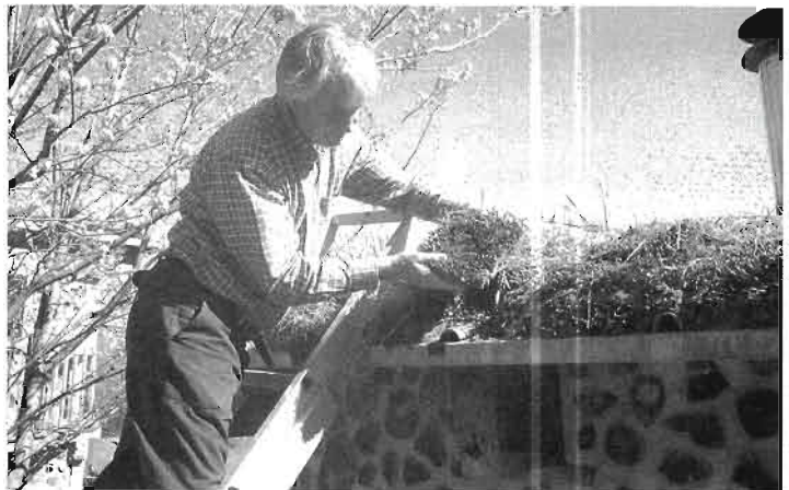
Fig. 8.16: The author installs a moss sod on the edge of the office roof.
