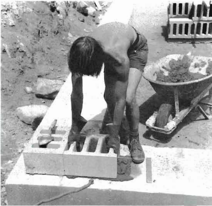
Fig. 5.3: The author lays the first blocks, in mortar, at Log End Cave, keeping blocks tight against each other.
