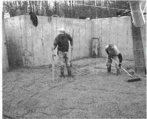
Fig. 4.14: The beam of a rotating laser level, 25 feet away, hits a grade stick. A benchmark on the grade stick shows if the concrete pad is high or low. Adding concrete or taking it away brings the pad to finished floor level.
