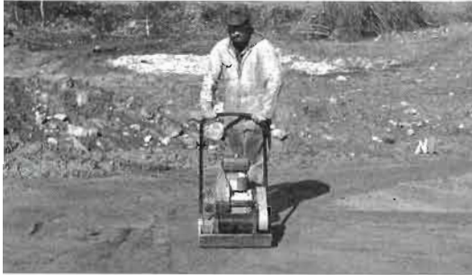
Fig. 3.4: Dennis Lee tamps the sand pad at Earthwood with a power compactor.
